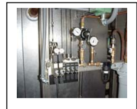
Pneumatic door control valves
