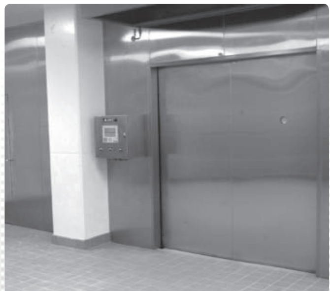
Horizontal sliding door autoclave installed at site.
